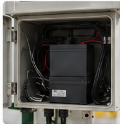
Secure Enclosure with Wiring
