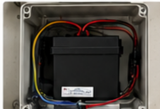
Secure Enclosure with Wiring
